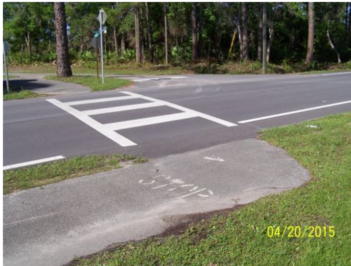
Crosswalk at the west end of the Bluff Road multi-use path, which lacks detectable warning surfaces.
