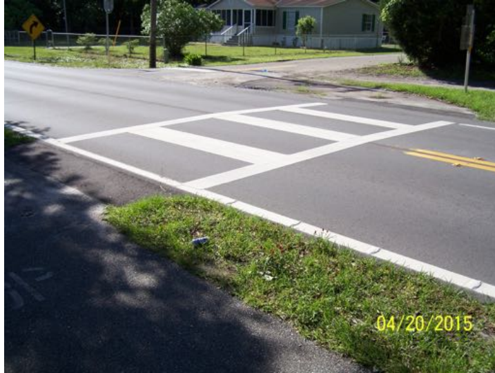
Crosswalk at the east end of the Bluff Road multi-use path, which lacks detectable warning surfaces.
