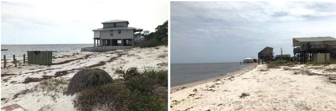
Figure 19. Typical beach condition to support a Type C Dune at end of Gulf Shore Boulevard near R-221 (left, view to the southwest, taken August 23, 2021) and vegetation only at Bald Point near R-231 (right, view to the southwest, taken August 24, 2021).
